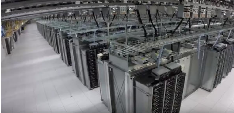
Figure 1.17: Large computer “server farm.”
