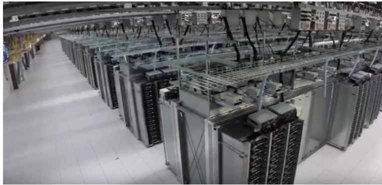
Figure 1.17: Large computer “server farm”.
