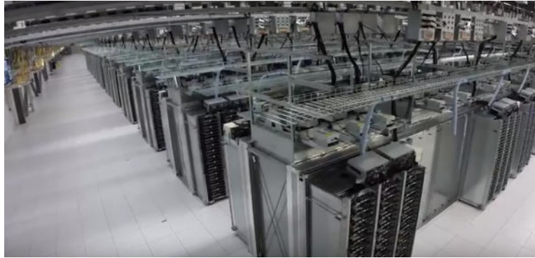
Figure 1.17: Large computer “server farm”.
