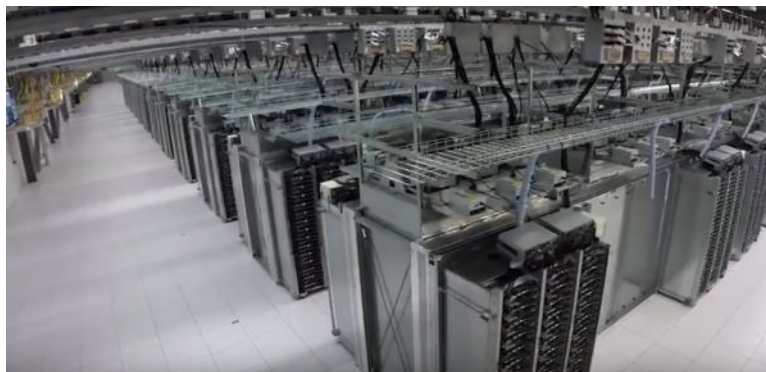
Figure 1.17: Large computer “server farm.”
