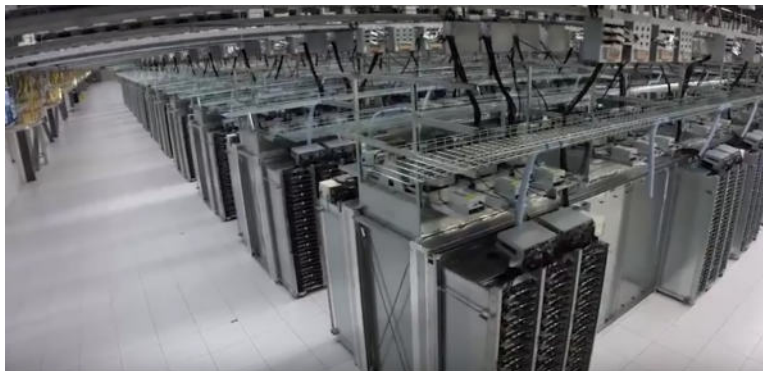
Figure 1.17: Large computer “server farm.”
