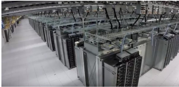
Figure 1.17: Large computer “server farm”.
