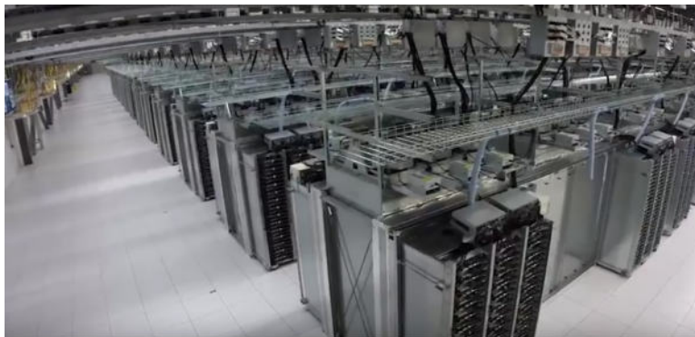
Figure 1.17: Large computer “server farm.”
