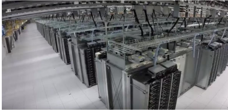
Figure 1.17: Large computer “server farm”.
