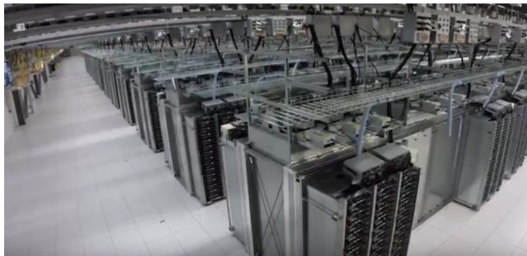
Figure 1.17: Large computer “server farm.”
