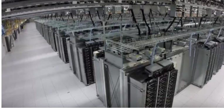
Figure 1.17: Large computer “server farm.”
